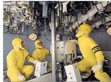
Maintenance work of control rod drive mechanism at the reactor lower head (Source: Chubu Electric Power Co.,Inc.)
