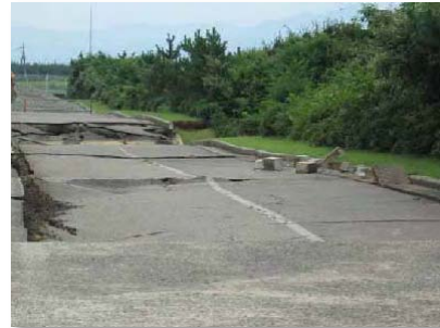
State of the on-site road of the Kashiwazaki Kariwa Nuclear Power Station after the earthquake (Source: TEPCO)
