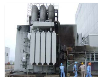
House transformer of Unit 3 after fire was extinguished (Source: TEPCO)
